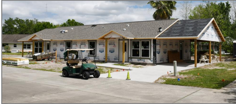
Progress on the new duplex. Needs completion of shingles, siding, painting, irrigation and landscaping as well as finishing the interior construction. Completion goal: Winter 2019
