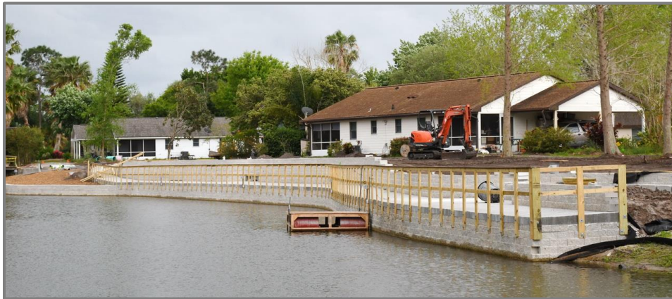
Lake wall construction. Needs completion of the sidewalks, light poles, irrigation and landscaping. Completion goal: June 2019
